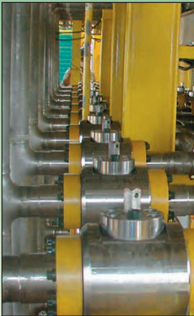
Manifold assembly prepared for actuator installation.
